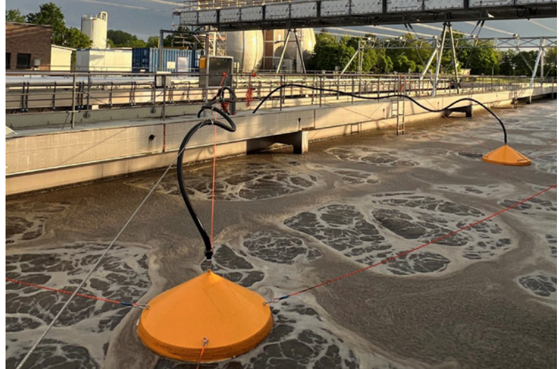
Figure 1: Setup of the EmiCo lite system at the investigated aeration tank.
