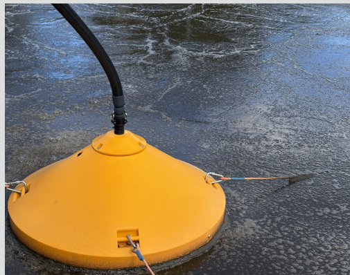
EmiCo lite at the aeration tank
